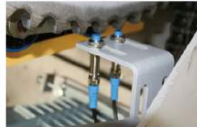
扶梯测速/扶梯防逆转 Main drive speed detect
