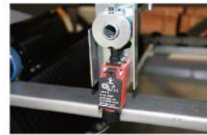
梯级塌陷 Step collapse detect
