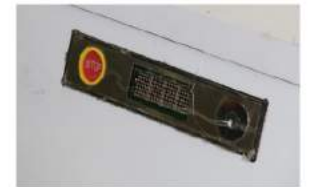
急停按钮 + 故障显示 Emergency stop button + fault display
