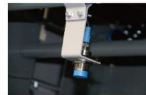
梯级丢失 Step missing detect
